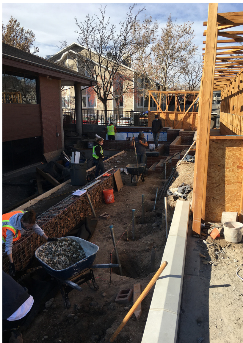
Student team (Nicole Lyman, Sydney Carillo, Derek Stephens, Zach Smith) and volunteer Carl Christiansen constructing a gabion retaining wall with donated recycled brick from HHI Corporation in Ogden.
