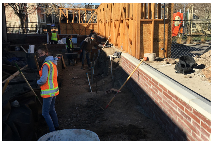
Nicole Lyman with new masonry retaining walls (a majority of masonry labor was donated by IMS Masonry).
