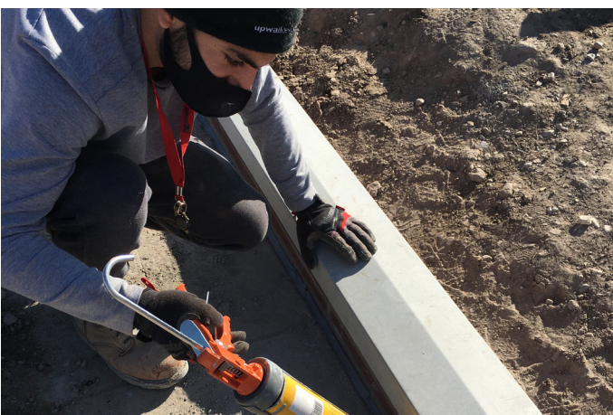
Attention to detail: Tigran Aganikian caulking a joint at a sidewalk edge.
